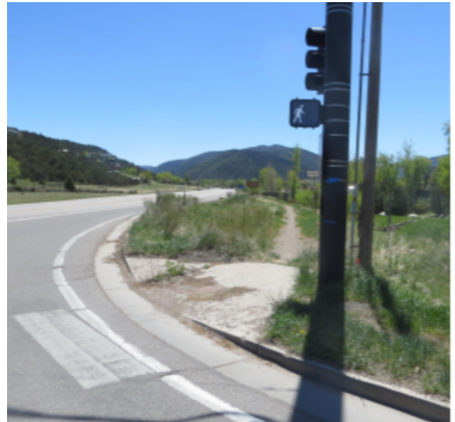
The unpaved “CDOT trail” on the west side of the CDOT SH 82 right-of-way, looking south from Original Road intersection. Photo: Eagle County
